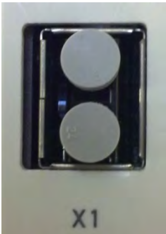
Figure: Blind plugs in unused sockets
