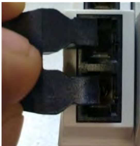
Figure: Blind plugs in unused sockets
